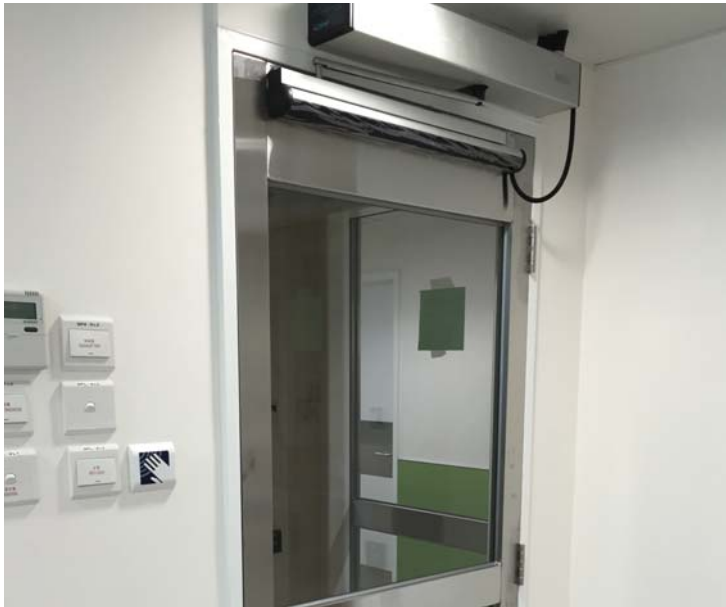
▲ Architectural Services Department Fanling Families Clinic FD20
