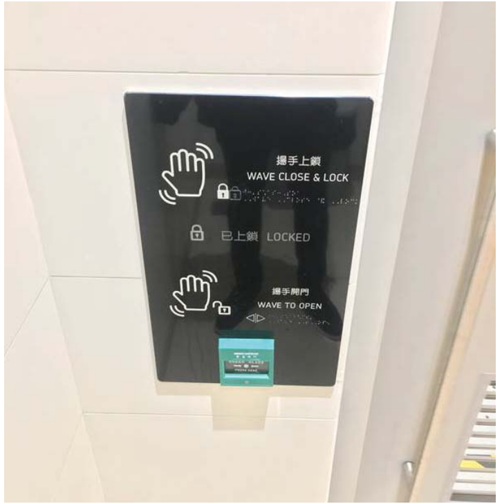
▲ Hong Kong Children's Hospital Barrier Free Access Solution with Sliding door Operator (Customized Panel)
