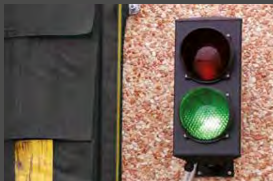
SEMAFORI TRAFFIC LIGHTS
